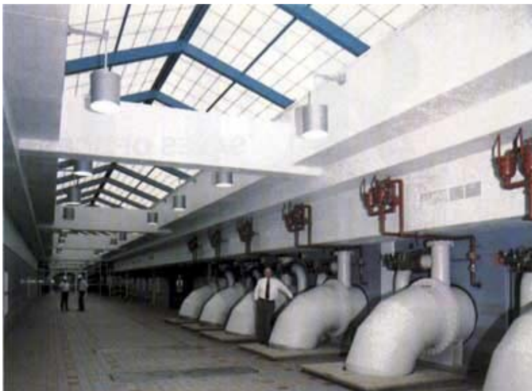
Huge pipelines transfer conventionally treated and filtered water to the carbon contactors for removal of organic contaminants.
