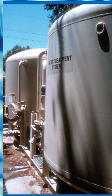
Carbon treatment vessels.
