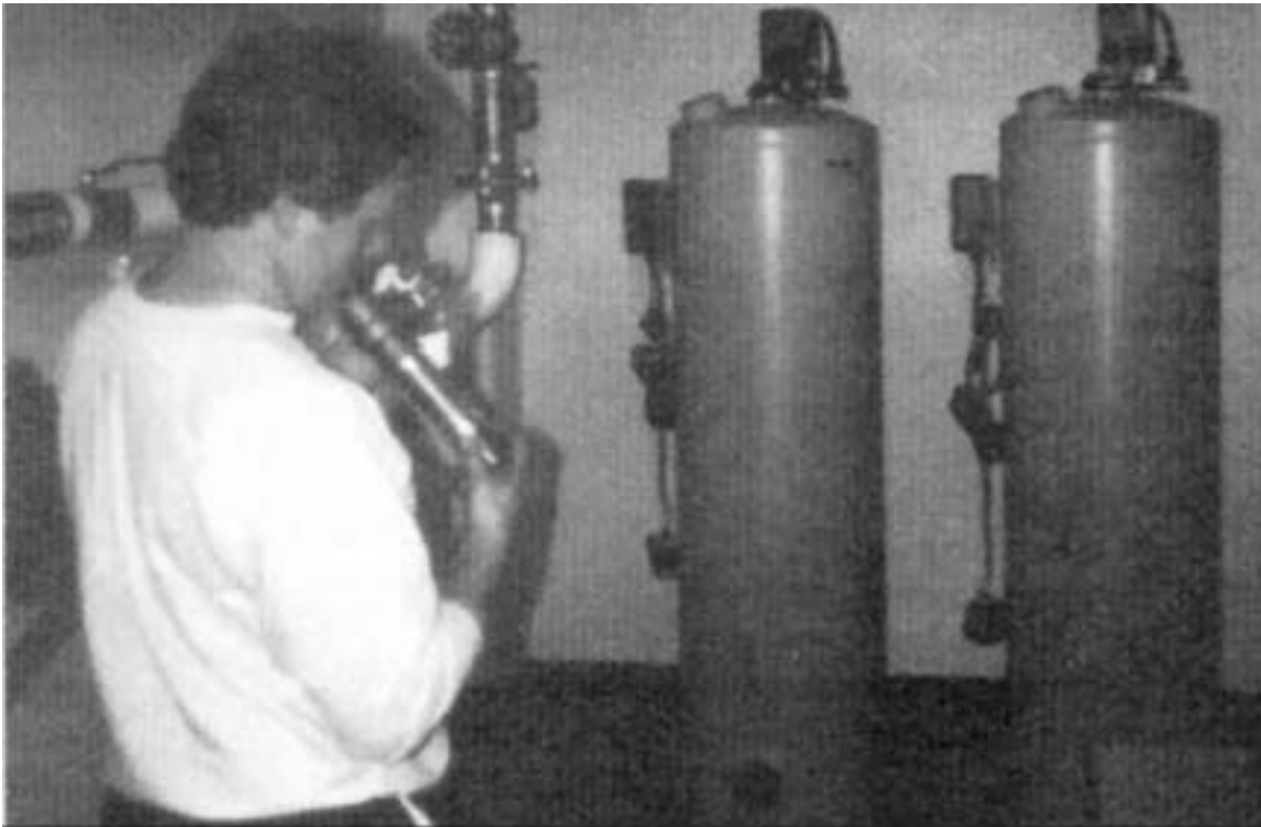
Ed Mohler, a master mechanic with Eichelberger's, Inc., Mechanicsburg, PA, prepares to work on a pair of carbon filters used for hydrogen sulfide removal.
