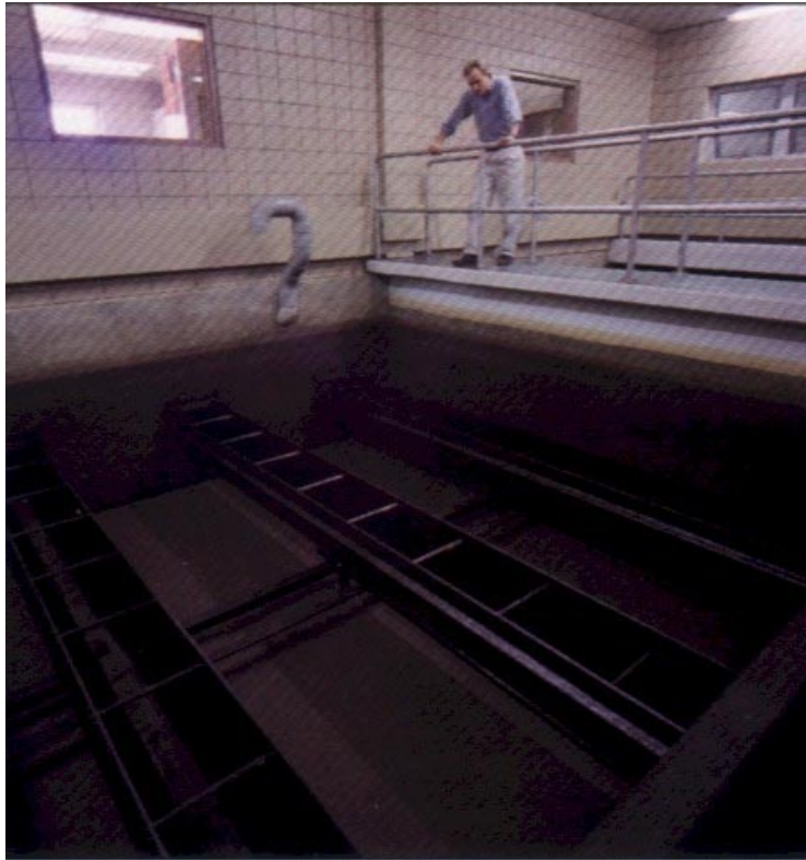
Pictured is one of five GAC filters that comprise the shallow bed system at the Robinson Township, PA, Water Treatment Plant.
