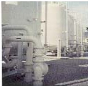
EFFECTIVE HYDROGEN SULFIDE REMOVAL FROM GROUNDWATER
